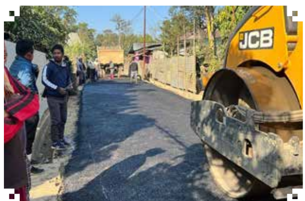
Inspection of black topping of road at Yurembam within Konthoujam AC and interacted with the people in the area
